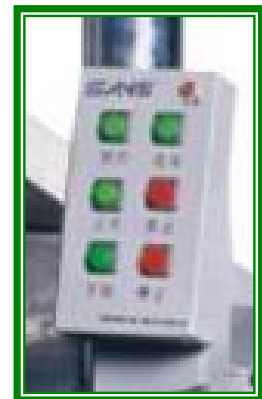
Fig2. Operation control panel
